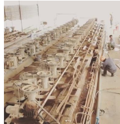
Fluorspar flotation plant
